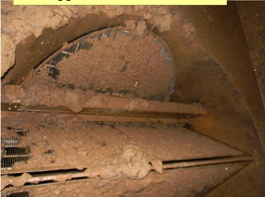
Plugged Screens at outlet
